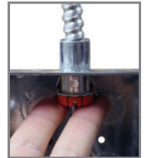
Push fitting and conduit back thru knockout
